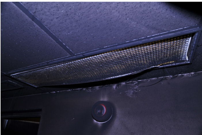
Photo 5 – Neighbouring light fitting showing diffuser in place
