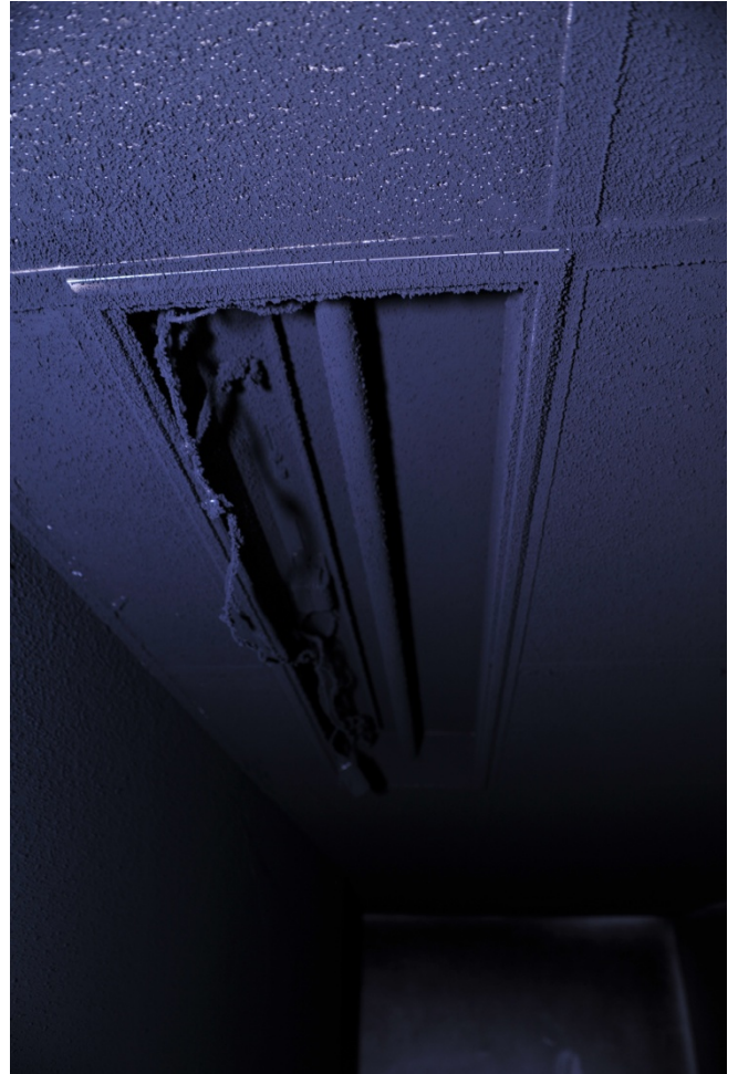
Photo 4 – Light fitting above seat of fire showing heavy sooty deposits
